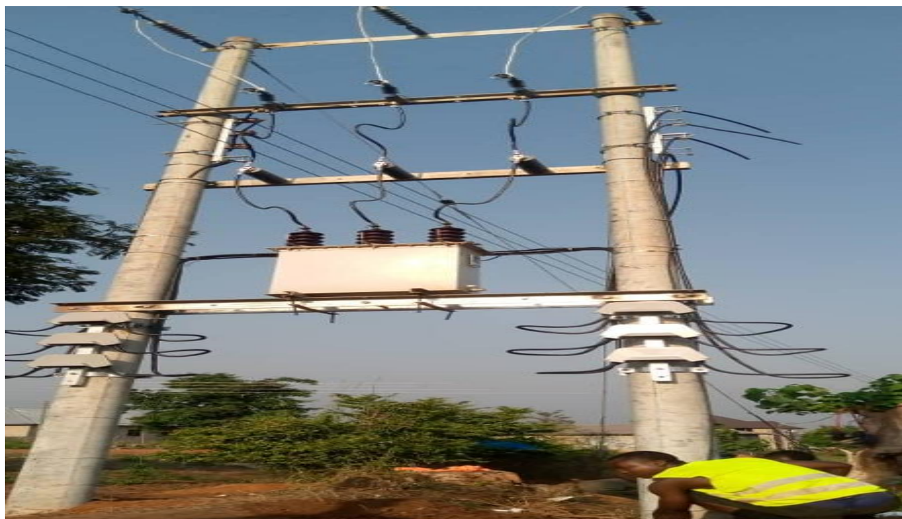
Rural Electrification Network
