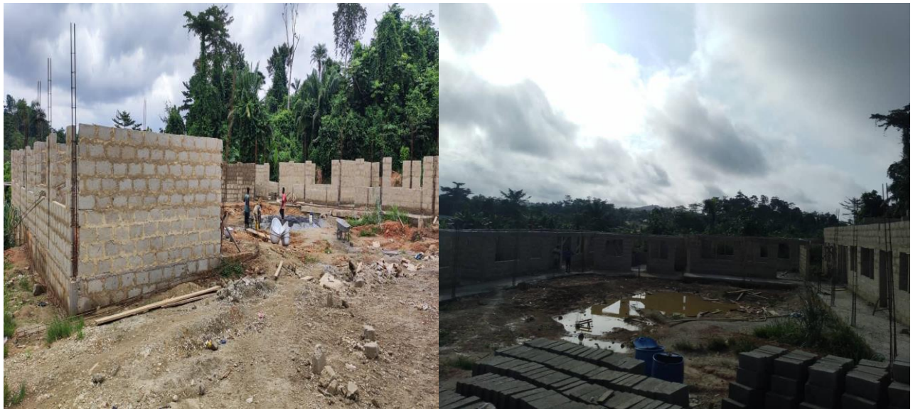
Began the Construction of 1No. 6Unit Classroom Block with Ancillary Facility At Dwirigum
