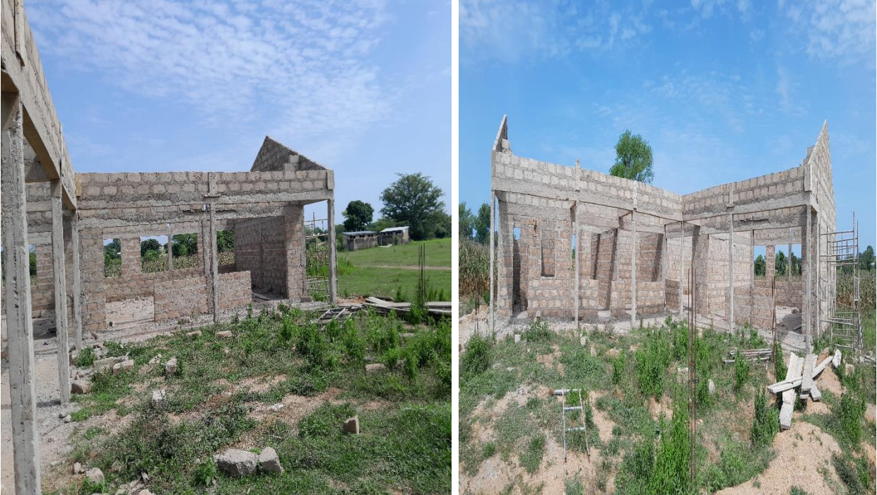
Constructed 1no. 2unit KG blocks supply 60no. Chairs with 6no. Hexagonal tables at Nyorkokor
