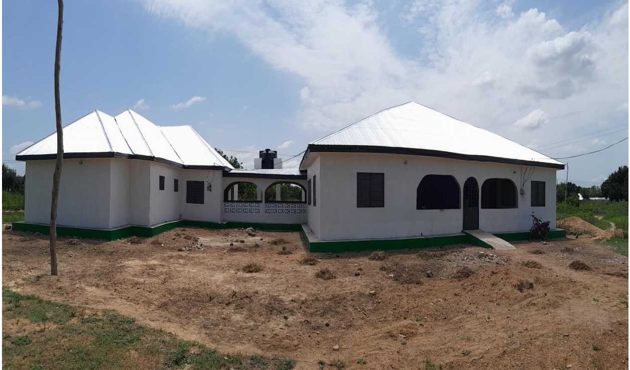
Completed the construction of 1no. CHPS compounds, drilled and mechanized 1no. Borehole and supply assorted medical equipment at Yipaala
