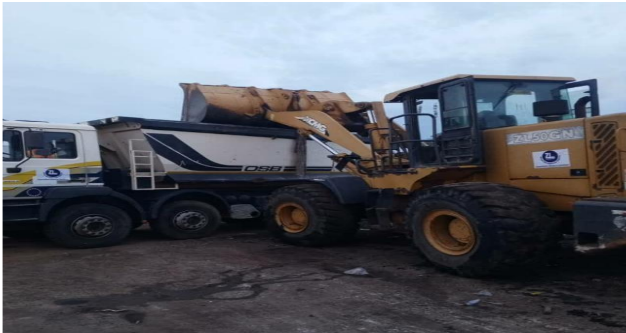
Evacuated Refuse Heap at Bazua Market
