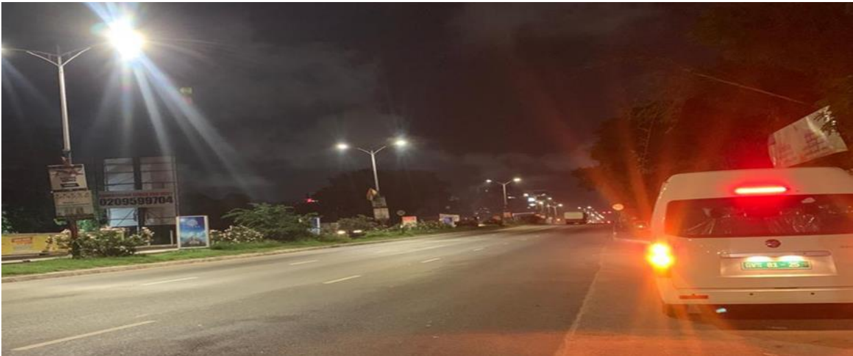
Picture 5: Installed 100 streetlights and maintained 200 on selected roads in the Municipality.
