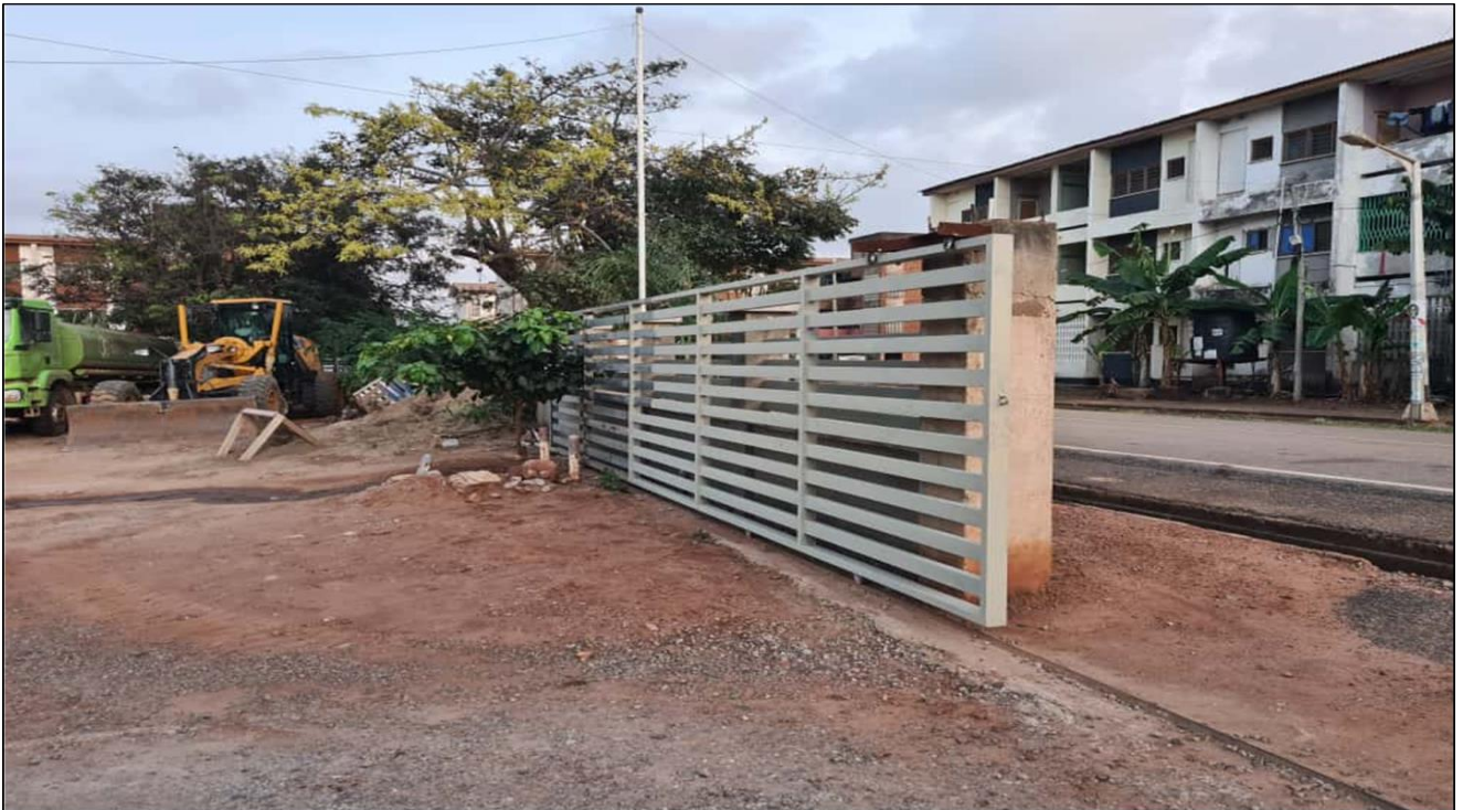
CONSTRUCTED PROPOSED FENCE WALL AND SECURITY POST AROUND ADMA MAIN OFFICE - SSNIT FLATS, ADENTA.
