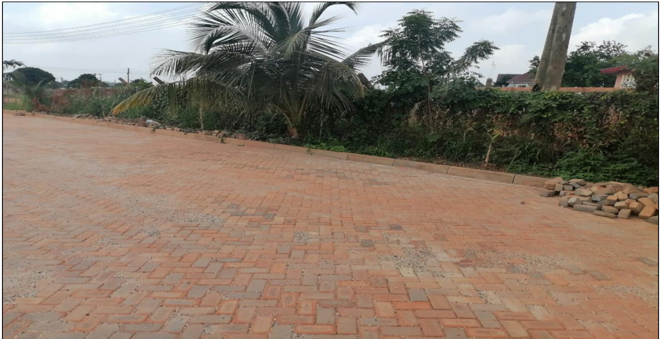
LANDSCAPING AND PAVING WORKS FOR FISH FOR DEVELOPMENT PROJECT SITE (FIDEP) AT AMRAHIA - ADMA
