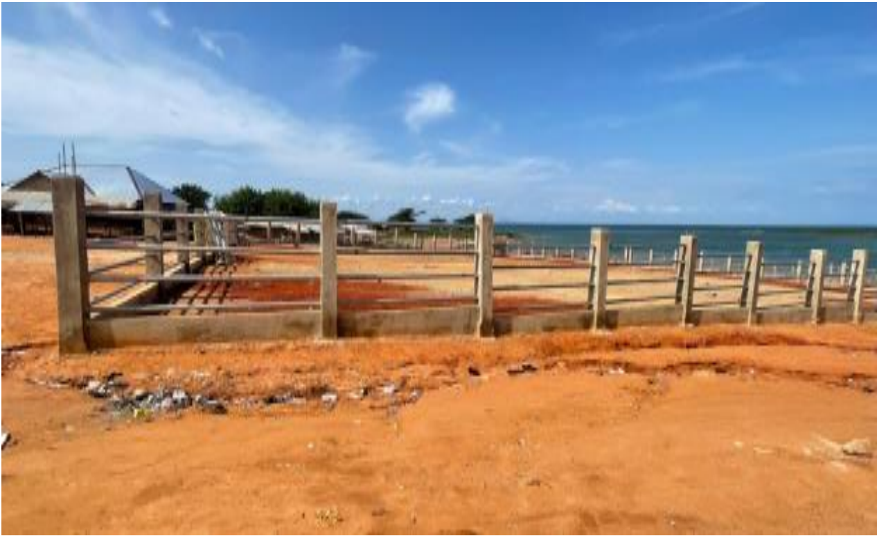
Constructed Galvanized Fence Wall of 40 × 40 Meters at Tulaku Livestock Market at Akateng
