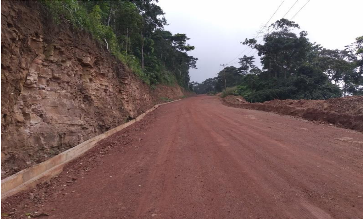
ESTABLISHED INDUSTRIAL SITE (GRADING OF THE AREA, EXTENSION OF ELECTRICITY, ACCESS ROAD AND WATER) AT BEPONG
