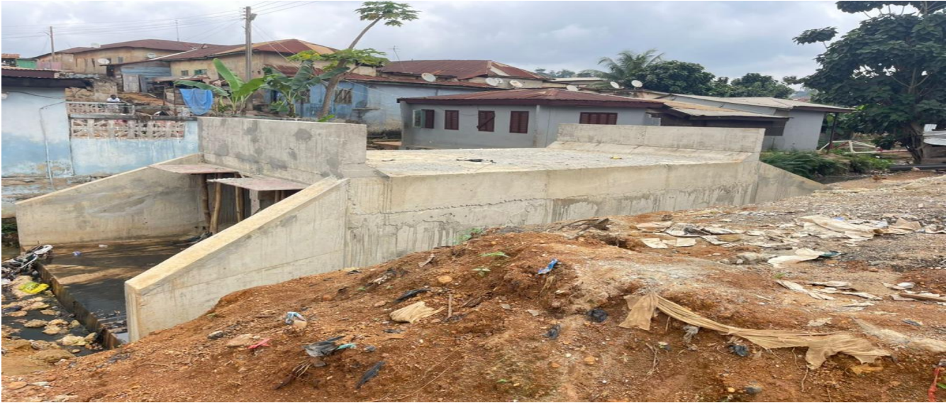
80 percent work completed on the construction of 2M x 2M double box culvert at Tutuka Tiatiaso.
