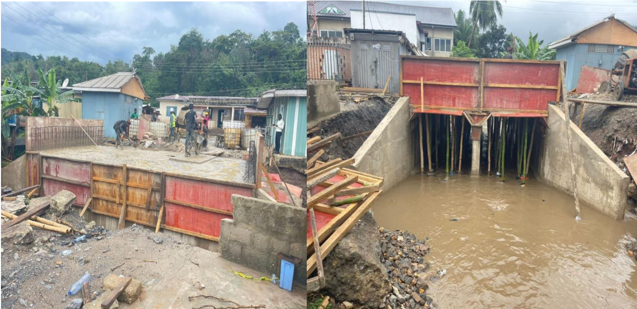
80 percent work completed on 2m x 2m double box culvert at Kwabrafosso.
