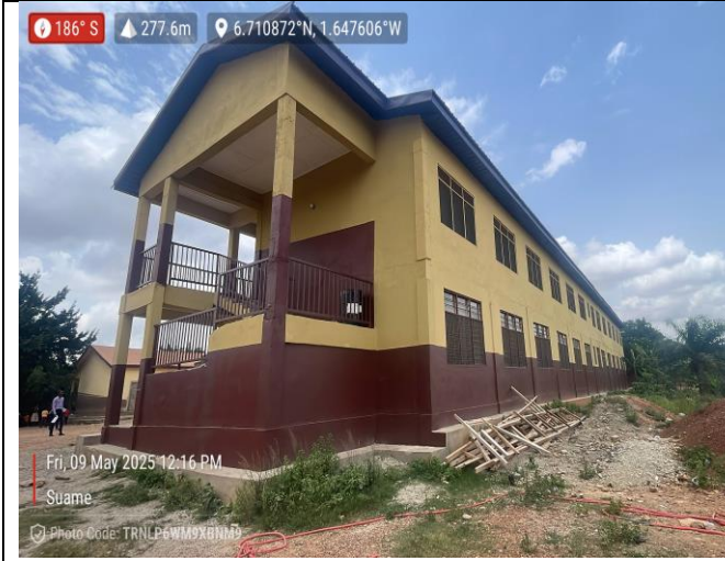
Constructed 1 No. 6 -unit Classroom Block at Adu-manu M/A Primary school (Phase II)
