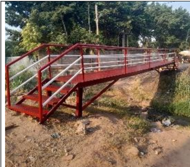
4 No Metal Foot Bridges Constructed at Atasemanso, Amankwatia, Duase and Moshie Zongo – (IGF)
