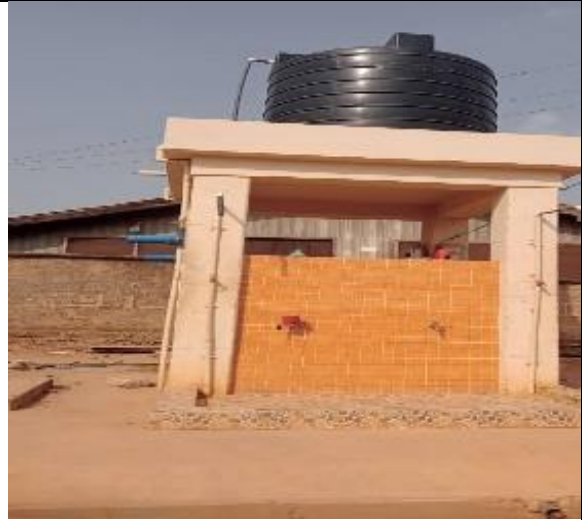
Constructed Mechanized 4No Borehole at Daban, Kokoso - Asubonteng, North Suntreso and Abrepo Mpatsie
