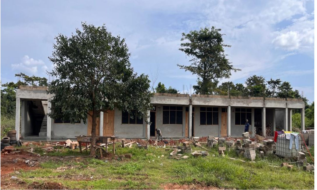
Construction of Single Storey Dormitory Block at Dadiesoaba Nursing and Midwifery Training School
