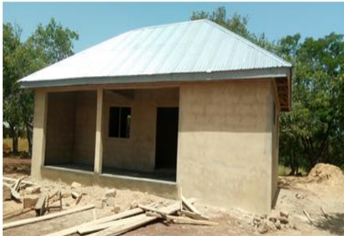
On-going construction of 1no. Staff Common Room with Store at Mary Immaculate R/C Primary School, Duotang (MP Initiative)
