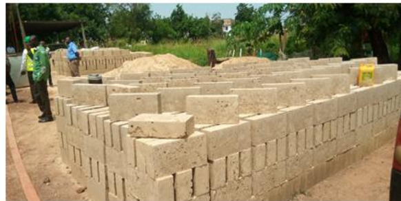
On-going Construction and Furnishing of 1no. 2-Units office for Ambulance Service (DACF-Assembly)
