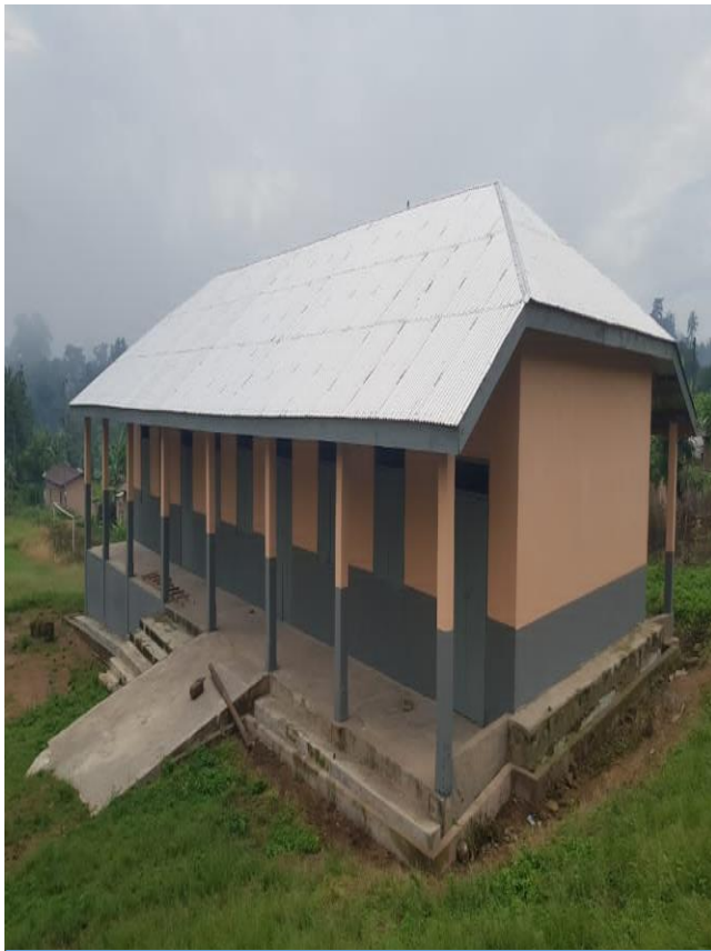
Rehabilitated a 3-unit classroom block at Santrokofi Gbodome D. A Prim. School
