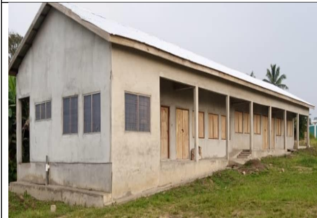
Completion of 1No. 3-Unit Classroom Block, Urinal, KVIP and Office at Kwahu Tafo. (85% Completed)
