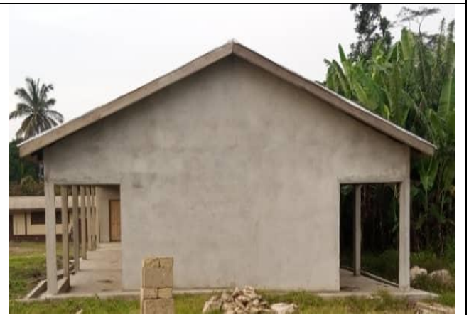
Completion of 1No. 3-Unit Classroom Block, Urinal, KVIP and Office at Kwahu Tafo. (85% Completed)
