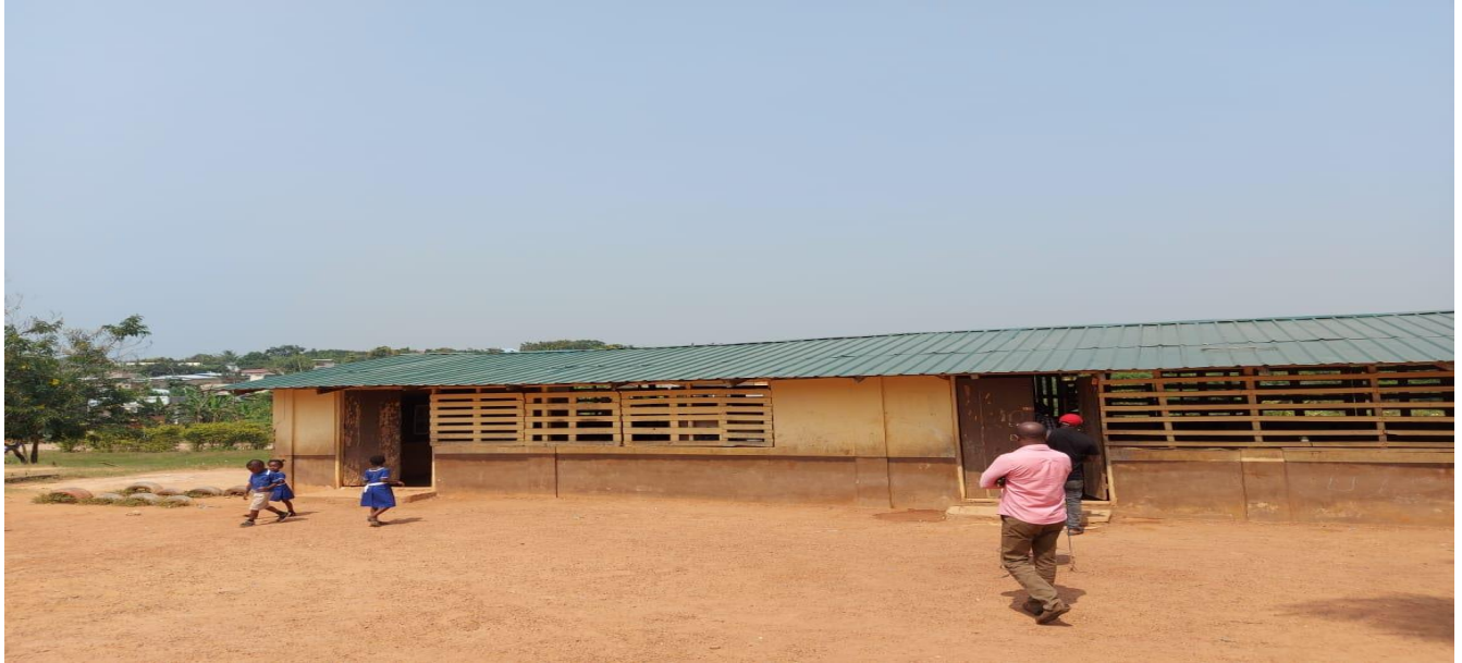
Damaged roof at St. Andrews Anglican M/A Basic School at Taido Completed – IGF
