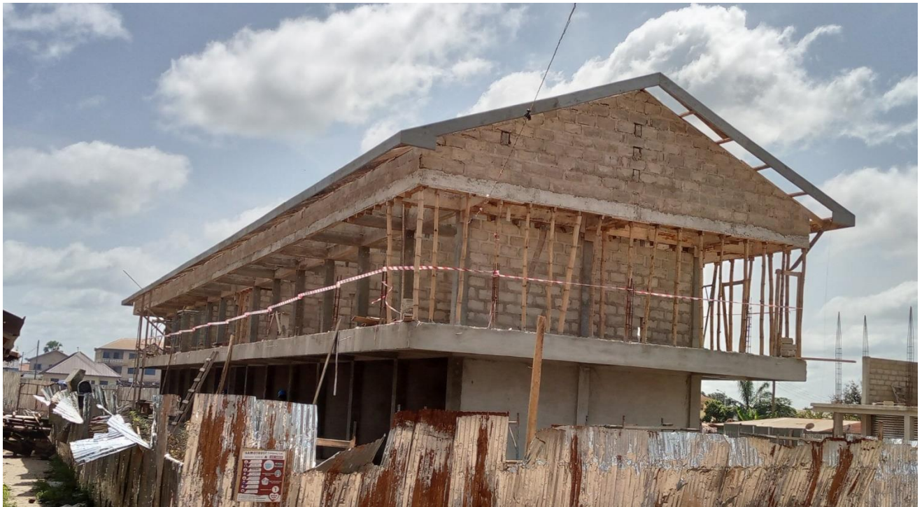
(Constructed 1No 48No. lockable stores and external works at Berekum Thursday Market) - GSCSP
