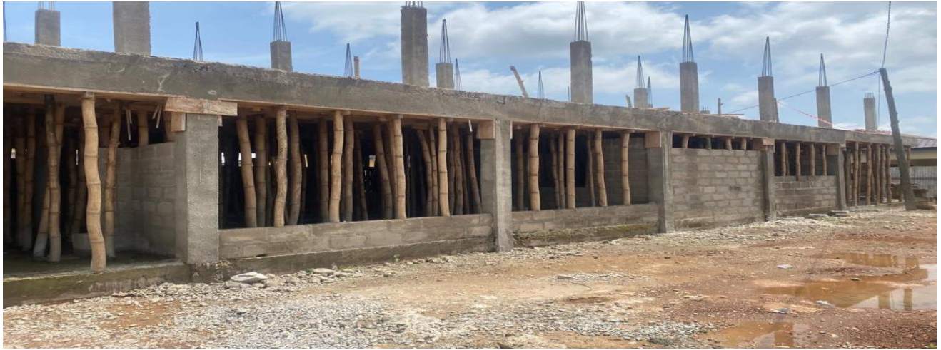
(Constructed 1No 40No. lockable stores, banking hall and external works at Berekum Thursday Market) - GSCSP
