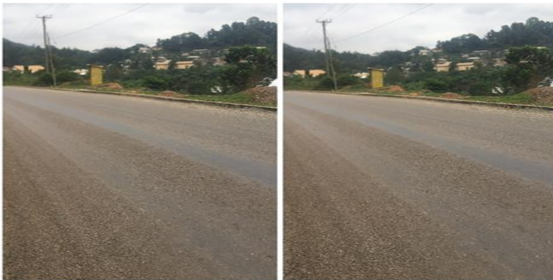
Rehabilitation of Mactina junction – Government Hill – Nyamebekyere with Primer and First Seal AC -10, Walkway, Covered u Drain, Road line Marking,
