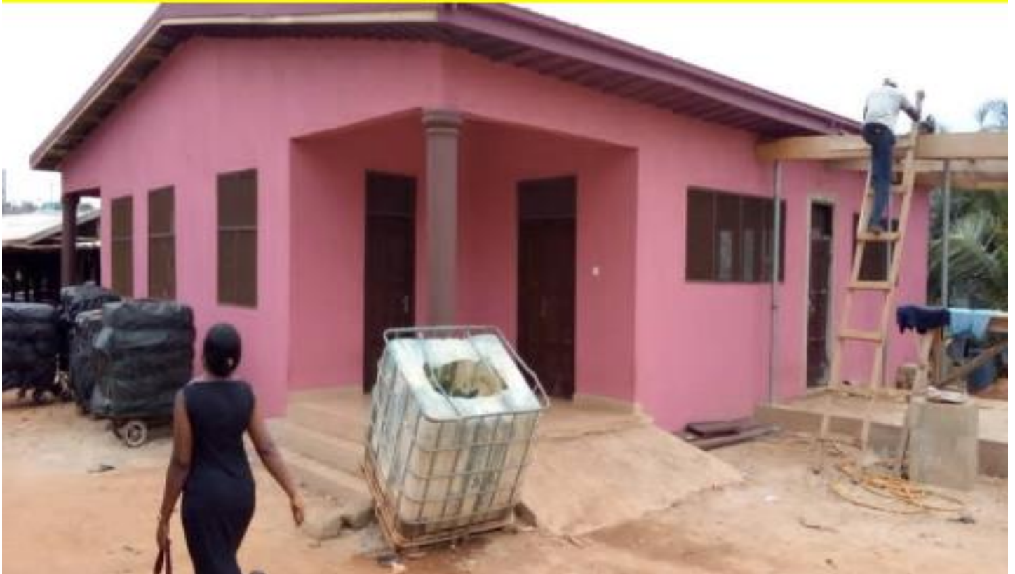
1NO. 3-UNIT ABATTOIR WITH SEWAGE CONTROL SYSTEM AND ANIMAL DRESSING OPEN SHED SOFOLINE-KWADASO CONSTRUCTED (DACF-RFG)
