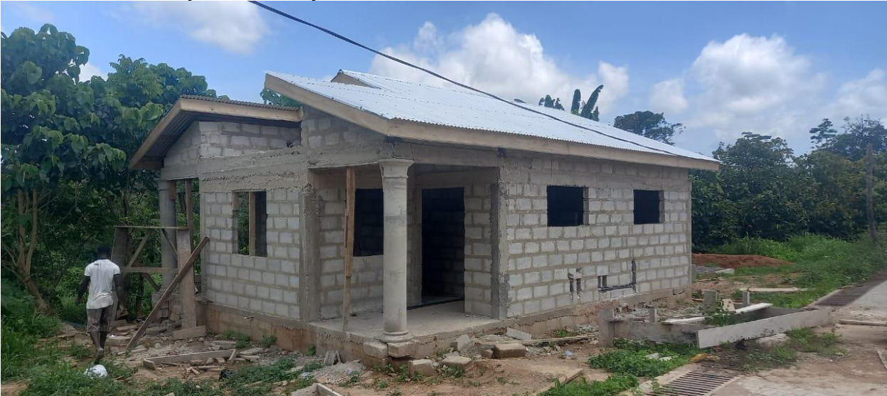
10-Seater Toilet Facility at Asiwa Lorry Park
