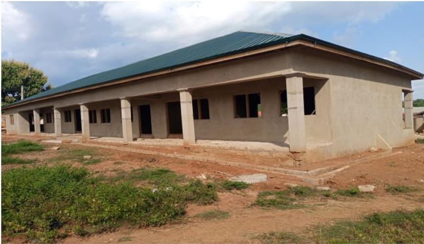
Construction and Furnishing of 1No. 3-Unit Classroom Block, Office, Store and Staff Common Room at Pokukrom Ibrahimyya Islamic School (Funded by: DACF)
