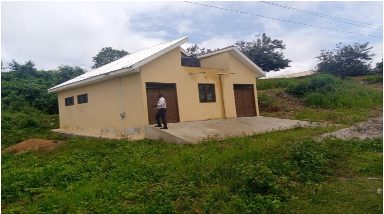
Constructed 1 no. 12 Seater WC Toilet With Mechanized Borehole And 3000 liters capacity Overhead Tank. At Agogooso(DACF -RFG)
