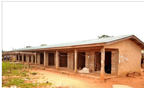
5. Ongoing construction of 10-unit lockable market stores from IGF at Bumbula Market
