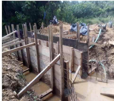
12. Continued the construction of 1 Single and 1 Double Cell Box Culvert at Ayensukrom No.2 Road
