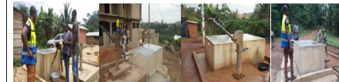
15. Constructed 8no. Iron and Manganese Removal Plant and Training for Water and Sanitation Management Teams at Prestea No. 3, Kwesikoko, Nyamebekyere, Cocoa Shed, Atobrakrom, Gambia (2no.) and Broni Nkwanta
