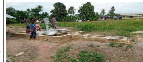
16. Drilled and Constructed 3no. Handpump Boreholes for K. Gyesei, Akotom and Huniso
