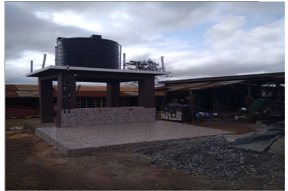
Figure 5: Mechanized Borehole With An Overhead Tank at Boukrom
