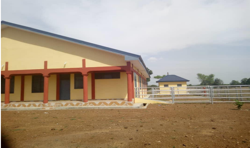
Construction of abattoir with Krall, biogas digester and a mechanized borehole at Yorogo
