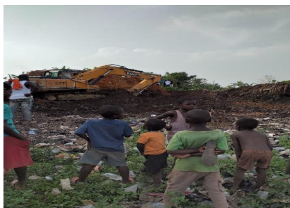
EVACUATION OF REFUSE DUMP AT SAMBRONUM THREE SITE AND DWENEWOHO ONE SITE
