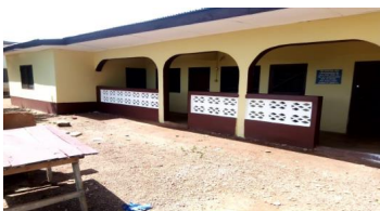
REHABILITATION OF SIX (6) BEDROOMS TEACHERS QUARTERS WITH HALL AT ASUADEI. THIS WAS CONSTRUCTED WITH
