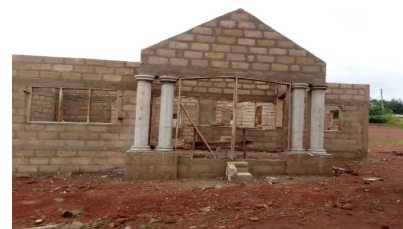
CONSTRUCTION OF MATERNITY BLOCK WITH OFFICE, CHANGING ROOM, STORE, ANC, DELIVERY ROOM AND LAY-IN-WARD AT POKUKROM
