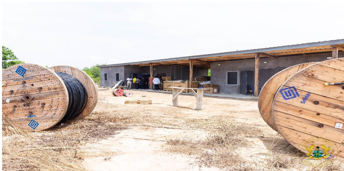
Alorkpem Power House
